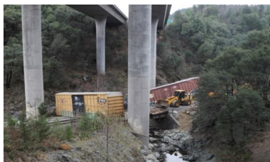
Figure 4 Union Pacific Train Derailment at I-5 in Shasta County, 2014.
