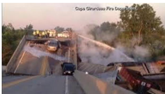
Figure 3 Union Pacific train derailment highway bridge collapse, Missouri, 2013.
