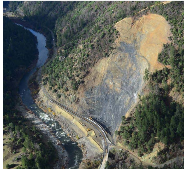
Figure 92. Landslide on Highway 299 near Big French Creek in Trinity County. Highway 299 was closed for several weeks to repair the road and construct a new catchment for future landslides (area between the slope and the road). Source: Caltrans 2018b.
