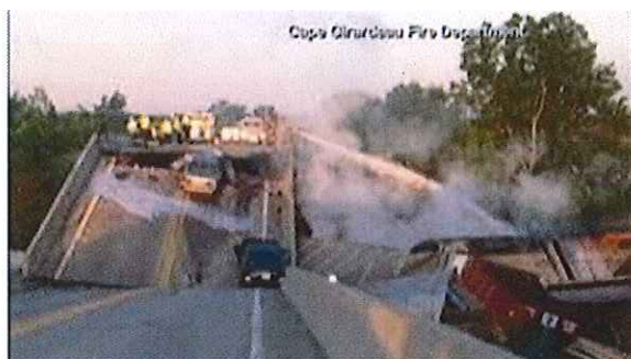
Union Pacific train derailment highway bridge collapse, Missouri, 2013.
